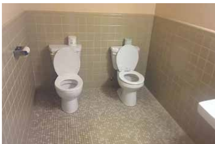
Figure 1: Wrong positions of two WCs within the same toilet
