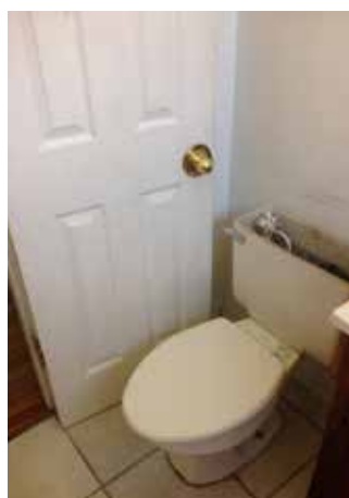
Figure 2: No space to open the door due to WC positioned in the entrance
